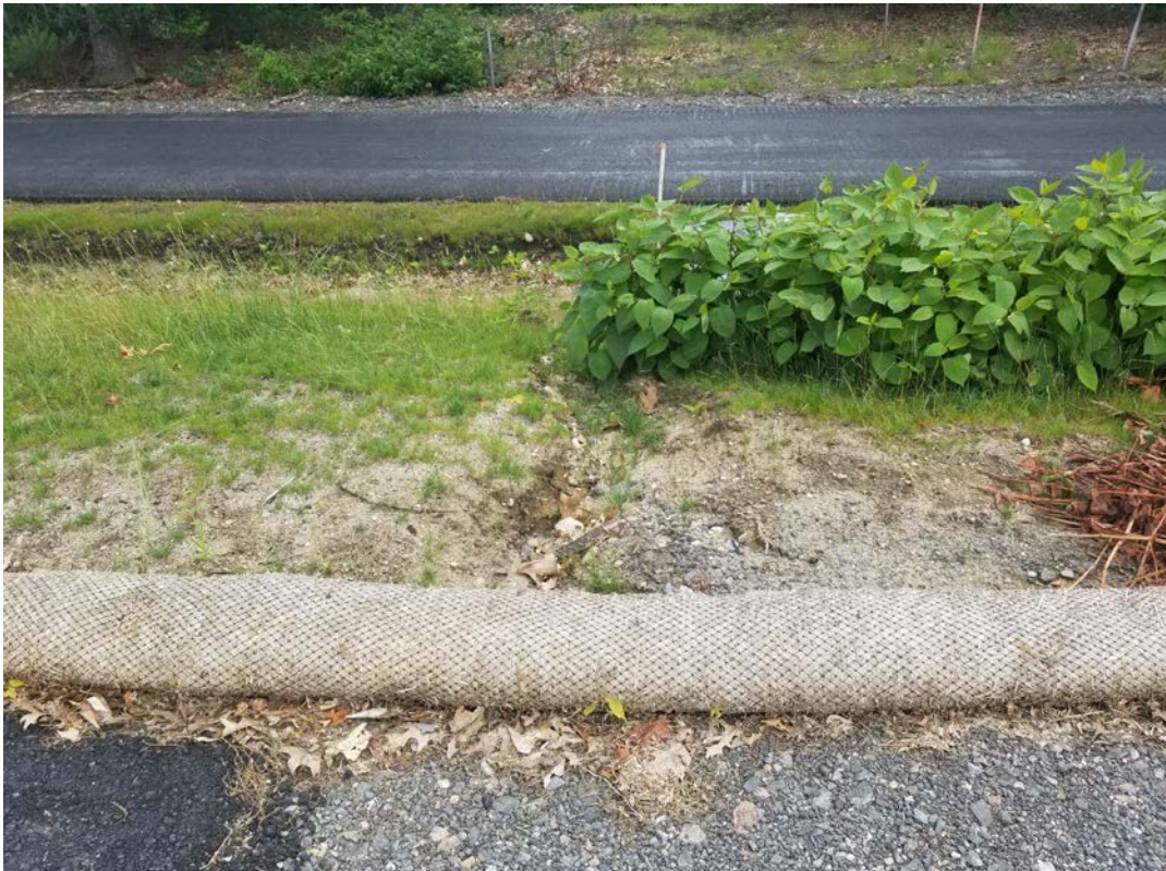
SLOPE AT COMMONWEALTH AVE TO BE FIXED
