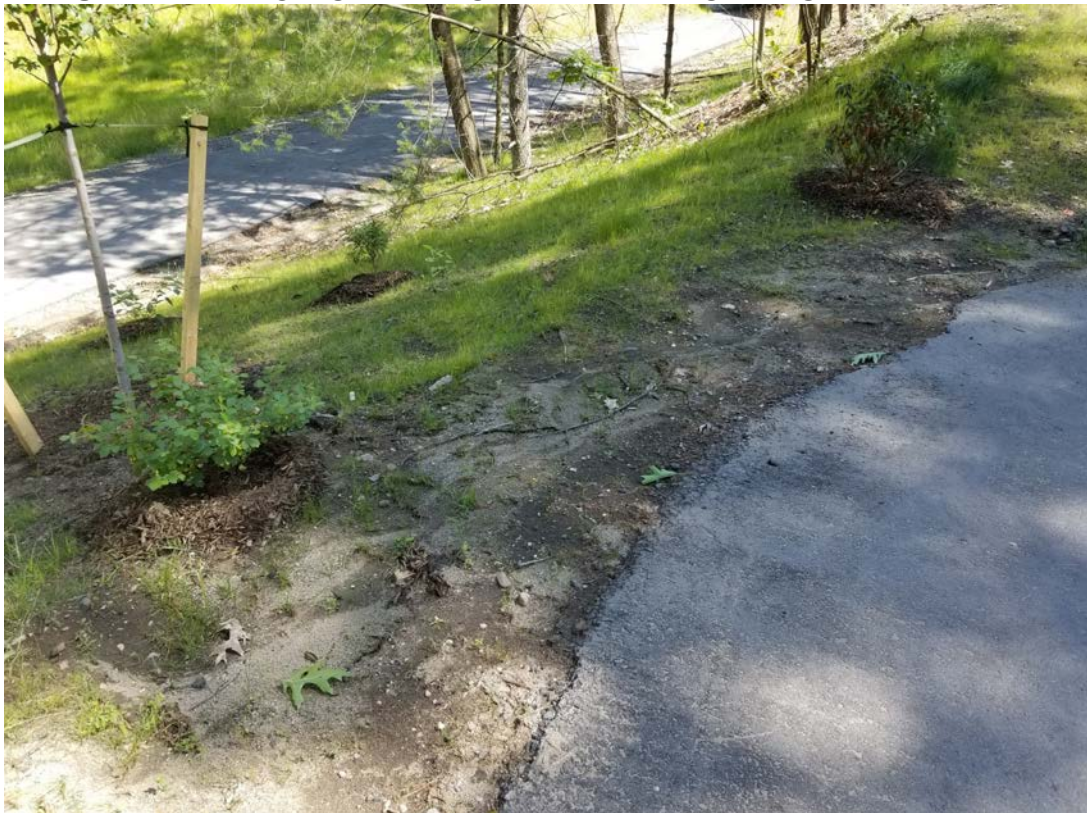
SEDIMENT RUN OFF AT POWDER MILL ROAD TO BE FIXED
