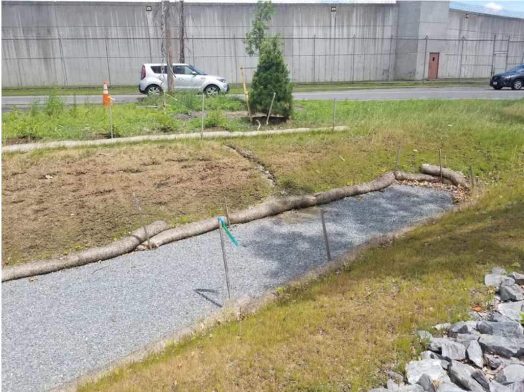
SLOPE AT COMMONWEALTH AVE TO BE FIXED
