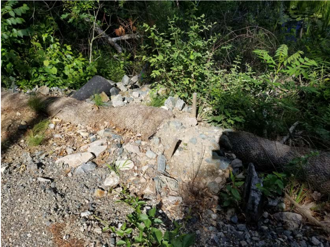
SEDIMENT TO BE REMOVED AND EROSION CONTROL TO BE PLACED
