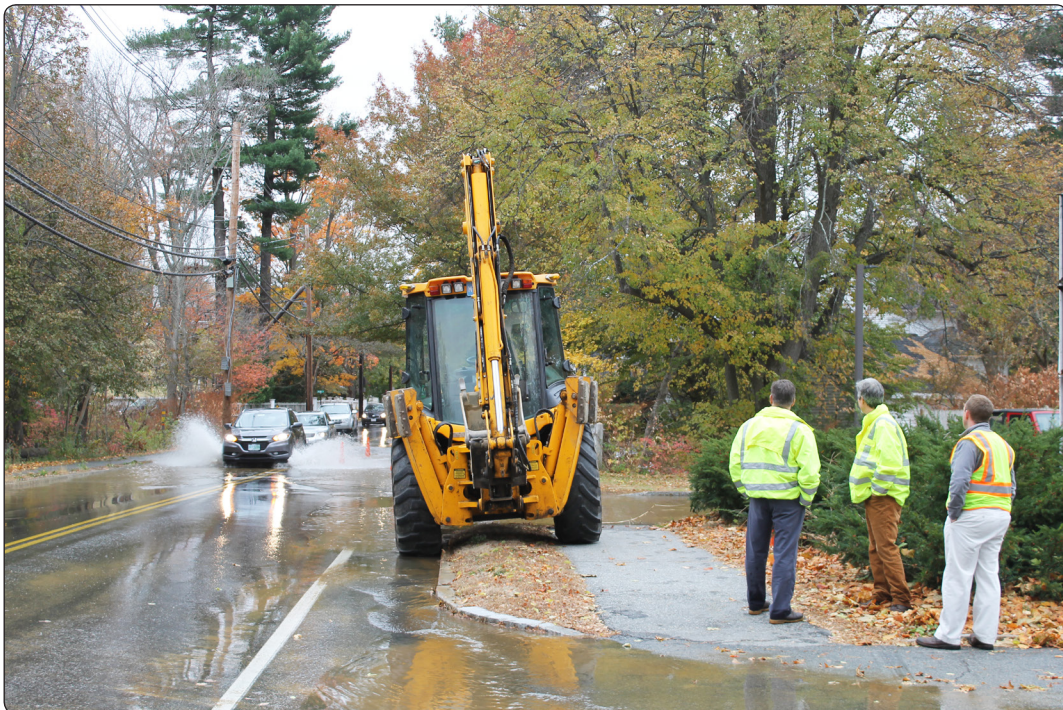
Water & Sewer Division responded to a water main break on Lowell Road on October 28.
