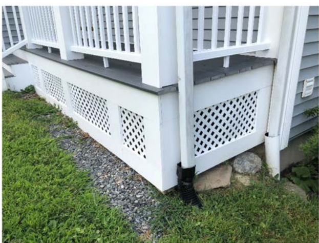
Roof Gutters Downspout Opportunity: Collect rainwater in a rain barrel or redirect into a rain garden
