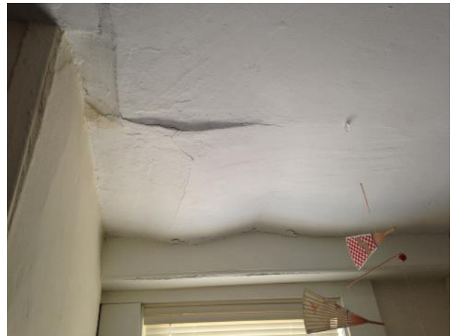
Figure 39: Area of detached plaster to the west of the chimney breast in Room 203.
