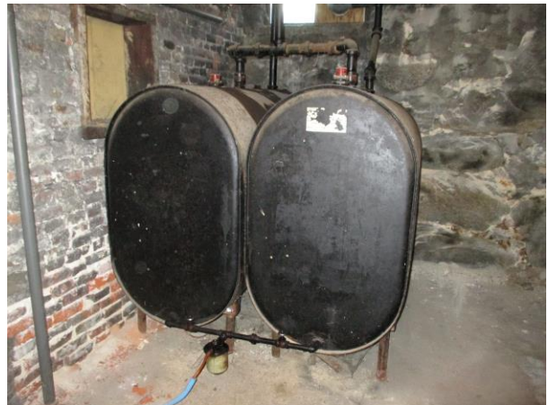
BAS: 4 Oil tanks on north wall
