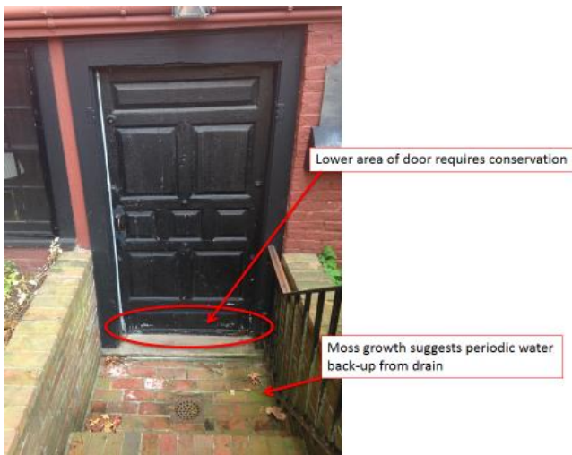
Figure 18: View of the historic Main Street bake shop entrance on the west elevation showing recessed entry, drainage problem, and rare eighteenth-century door.
