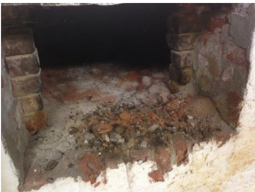
Figure 53: Accumulations of mortar, brick and creosote debris in the bake oven suggest interior flue deterioration.
