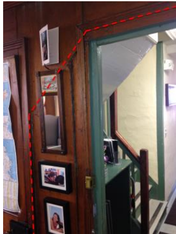
Figure 29: West wall of Room 104 showing alterations to woodwork to enclose what had originally been an open passage to 100b.
