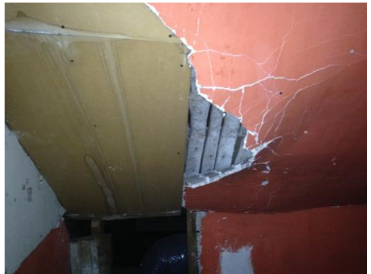
Figure 45: Ceiling plaster in Room 301 exhibits extensive collapse.
