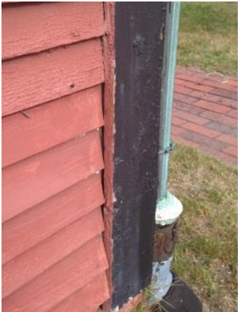
Figure 10: Northeast corner board showing deflection and protruding nails.
