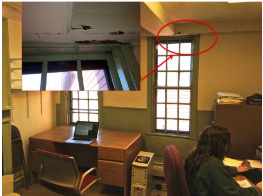
Figure 27: View of west wall, Room 103, showing localized paint and woodwork damage related to water infiltration from above. See also Figure 16.
