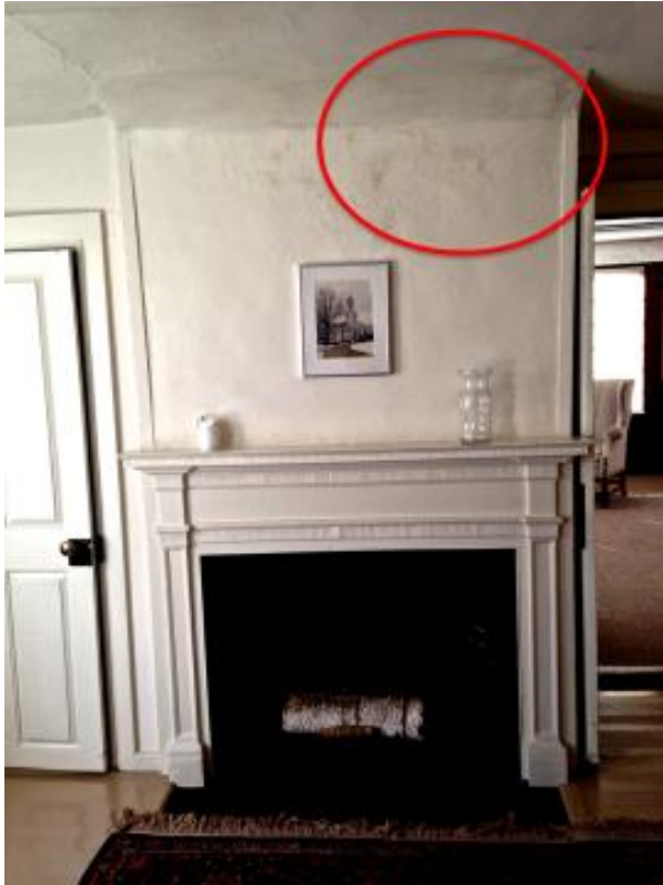
Figure 26: View of the fireplace wall in Room 102 showing the location of paint and plaster damage from chimney-related water infiltration.
