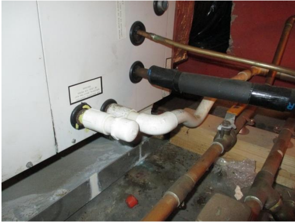
3rd: 6 Detail of southeast air handler
