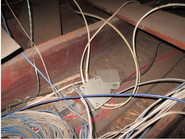
Attic: 1 Unsecured wiring west side.
