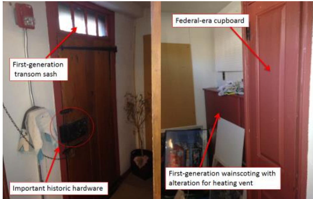
Figure 30: Room 107 architectural details. Left: North wall showing original details. Right: South wall showing original details and later alterations.
