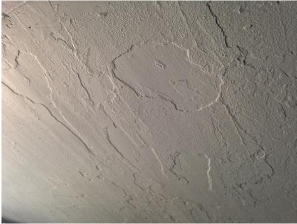
Figure 41: Paint failure in Room 209 related to poor adhesion over underlying calcimine.
