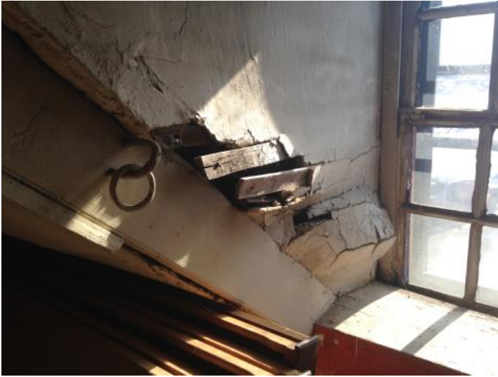
Figure 46: Surviving areas warrant immediate consolidation. Bulging plaster in dormer cheeks signals structural settling.
