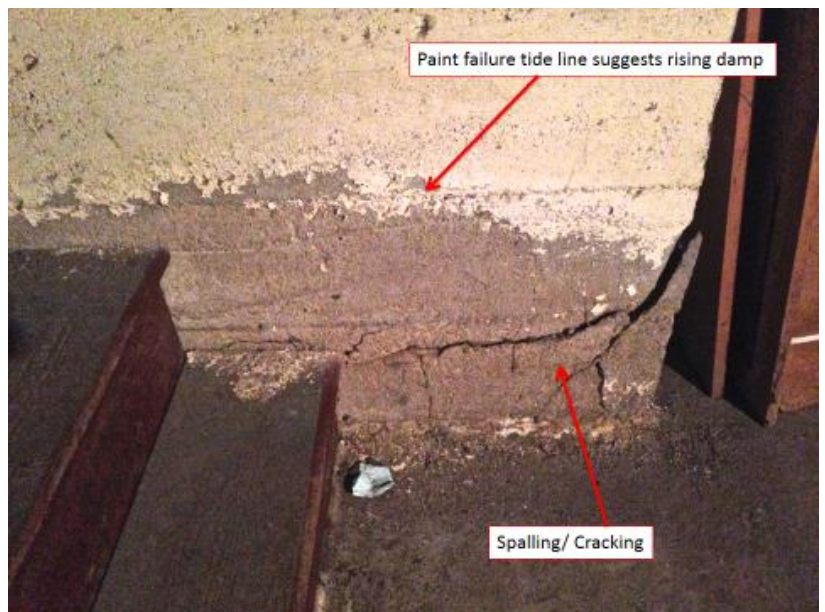
Figure 52: concrete delamination at the base of the main chimney suggests possible beginnings of rising damp.
