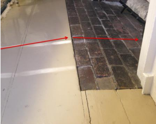
Figure 24: View of Room 101 floor and hearth showing deflection related to prior settling.
