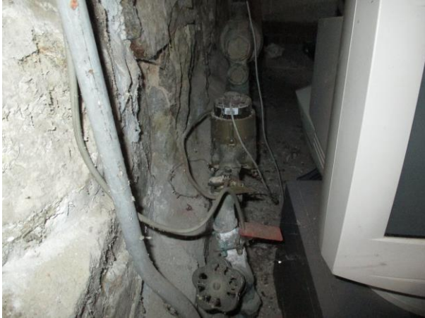
BAS: 1 Water line and ground wire, west wall.
