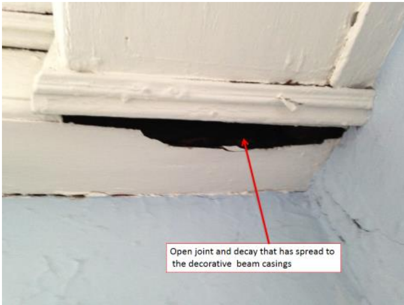
Figure 40: Front girt plate and girt intersection showing a spread-open joint and wood decay related to water infiltration.
