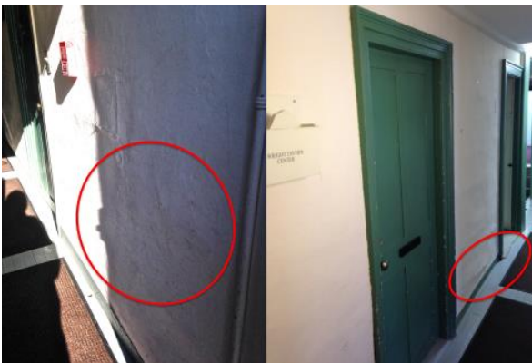
Figure 21: Two views of the east entrance hall looking west. Left: North wall near entrance. Right: South wall between doors to rooms 102 and 105. Red circles show the area of plaster to be consolidated.
