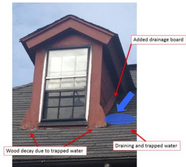
Figure 13: Northeast dormer showing water drainage, moisture trapped behind console foot, and wood rot.
