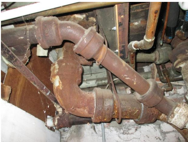
BAS: 16 Rusted cast iron drain line east center
