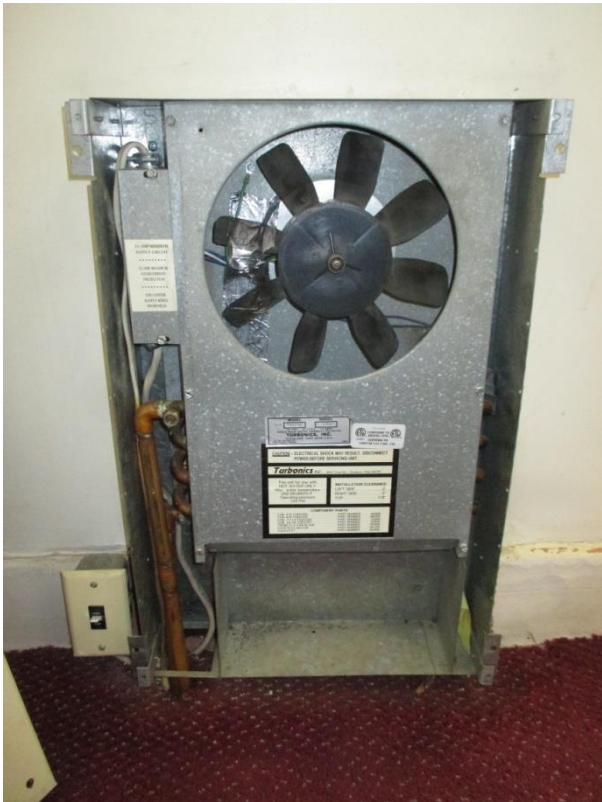
1 st : 1 Heating unit Room 100
