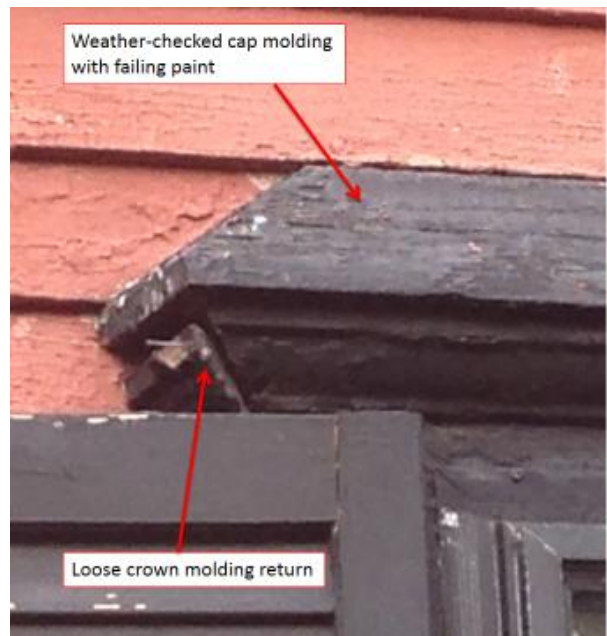
Figure 11: Detail of first-floor window on east elevation showing typical paint failure and deflected woodworking joints.
