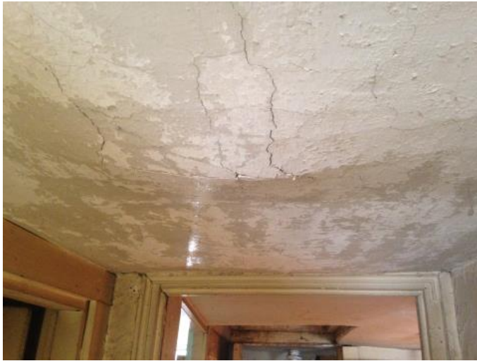
Figure 44: Failing ceiling plaster in 300c requires stabilization.
