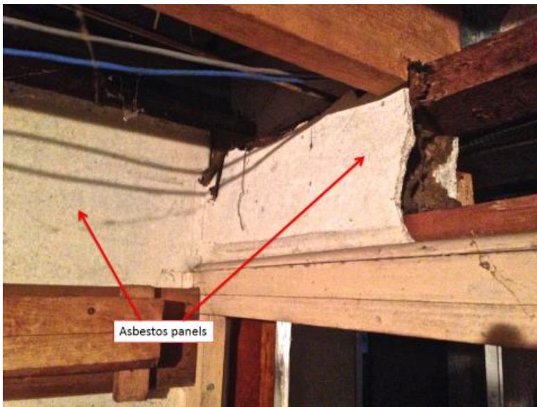
Figure 55: The small cold storage room below Room 101 is encased in asbestos panels that require abatement.
