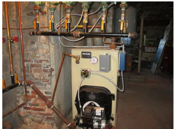
BAS: 5 Boiler in center of basement
