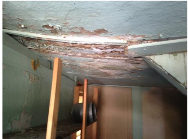
Figure 48: The ceiling and purlin post in Room 304 exhibit a pronounced sag related to past water leaks. The wood and plaster in this area are in danger of collapse.
