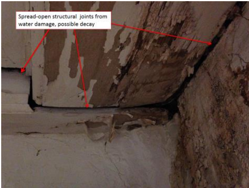
Figure 38: Intersection of the summer beam with the south girt, seen from inside the chimney closet in Room 203.
