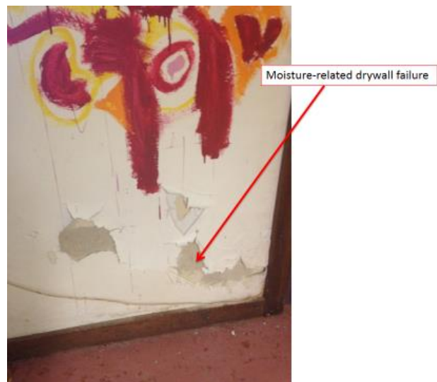
Figure 50: Failing drywall in the basement below Room 103, the result of high moisture levels, promotes mold growth.
