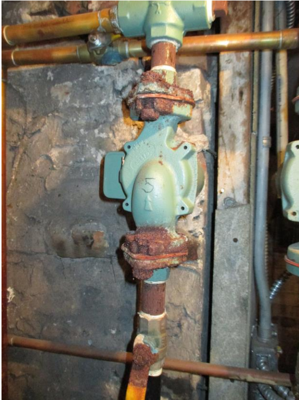
BAS: 6 Rusted valve above the boiler.
