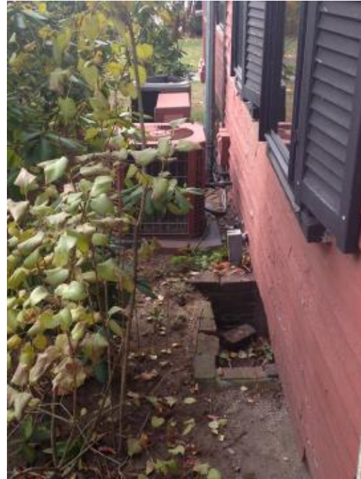
Figure 9: East elevation looking south, showing encroaching vegetation.
