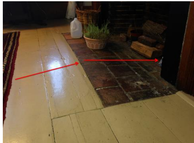
Figure 28: View of the fireplace hearth, Room 104, looking north, showing floor and hearth deflection.
