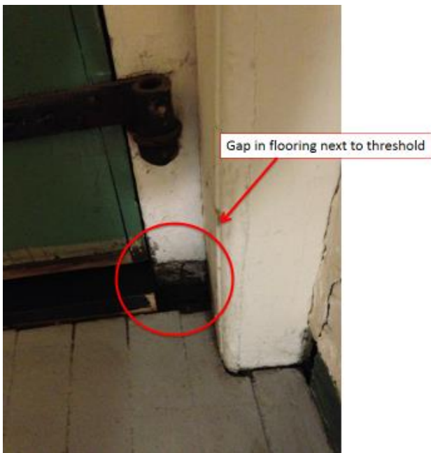
Figure 20: South end of east door threshold showing a gap that needs to be filled in.
