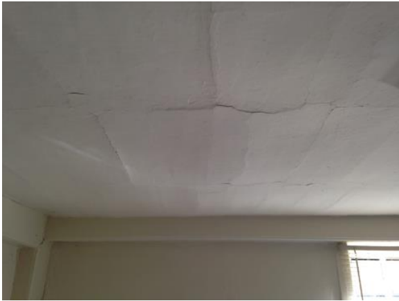
Figure 25: Ceiling, room 102, showing extensive cracking and detachment from lath.
