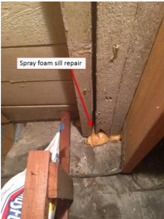
Figure 8: Detail of east foundation wall showing spray-foam repair
