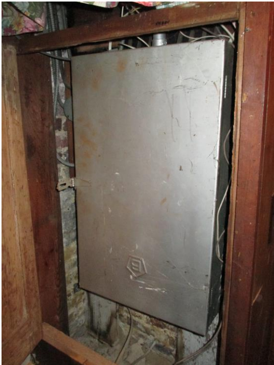
BAS: 11 Junction box in south room.
