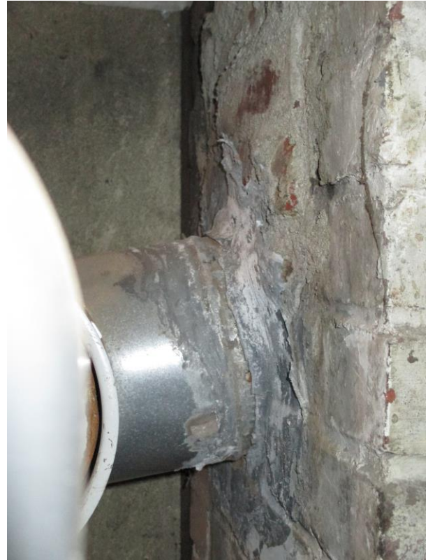
BAS: 8 Boiler vent
