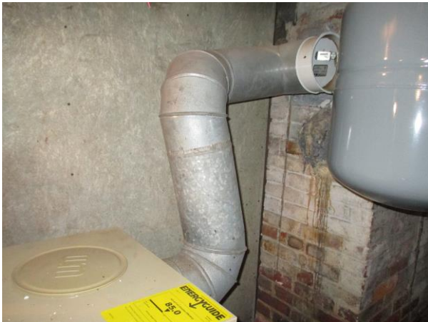
BAS: 7 Boiler vent
