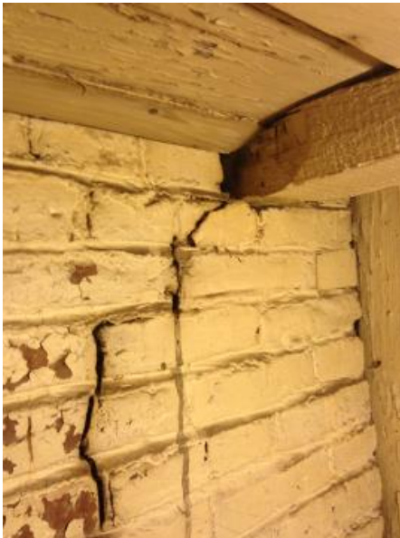
Figure 51: Settling crack in main chimney mass masonry as seen from the basement stairwell leading from Room 104.
