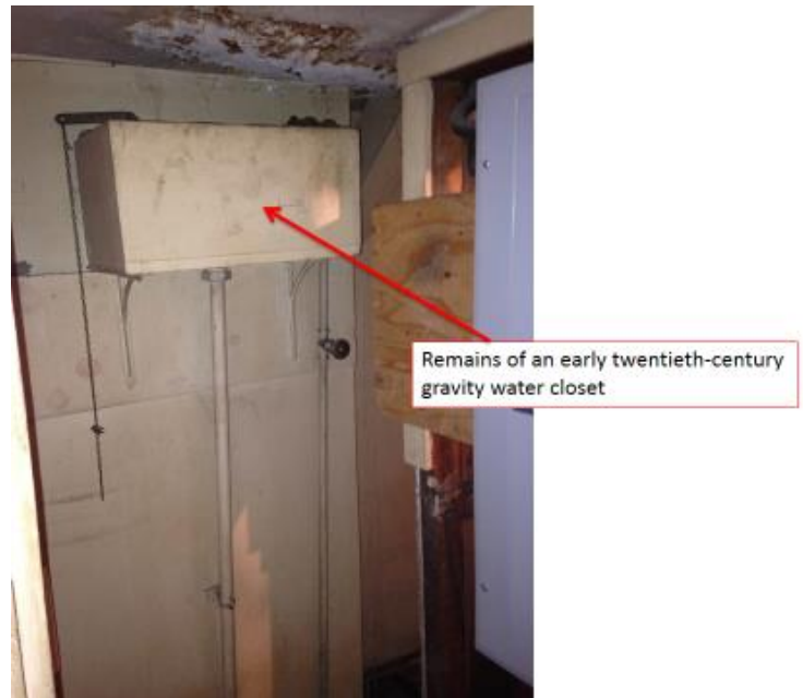
Figure 47: The east wall of Room 303 retains elements of an early twentieth-century water closet.
