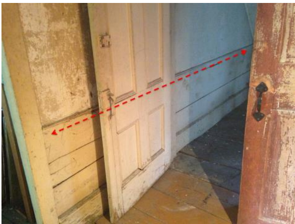
Figure 43: Continuous dado on south wall of 300a, passing behind a later wall partition, showing that 300b and 305 were originally a single space.
