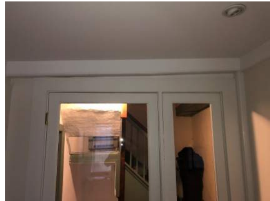
14) Sagging condition of timber girders typical throughout second floor ceiling.
