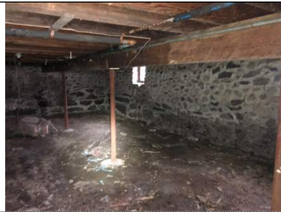
26) General first floor framing within area 3 and dirt floor crawl space, deteriorated lally columns.
