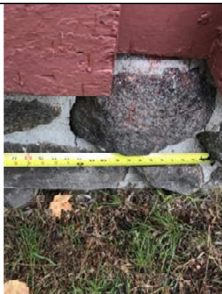
29) Exterior foundation of area 3 with visible crack.
