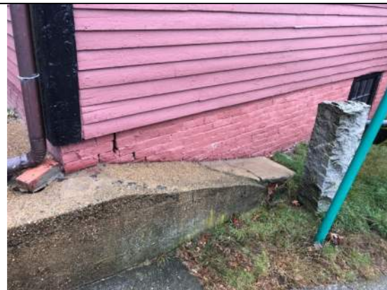
28) Exterior side of wall at photo 27, crack present.
