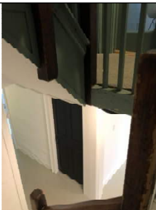
17) Continuation of center post through first floor level adjacent to bathroom door.
