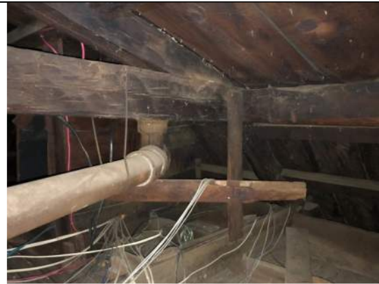
10) Sagging end of center girder at interface of hip roof at west side.
