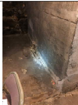
22) Spalling of interior concrete foundation at base in area 1.
