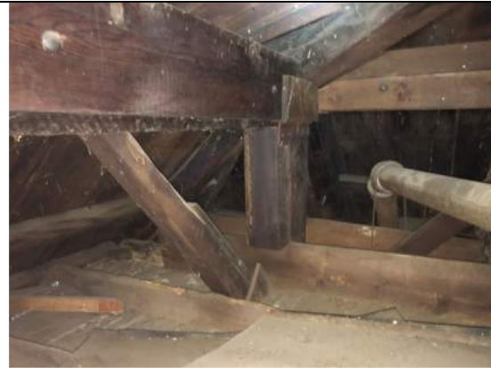
4) Typical hip post in attic above ceiling, typical of 4 locations.
