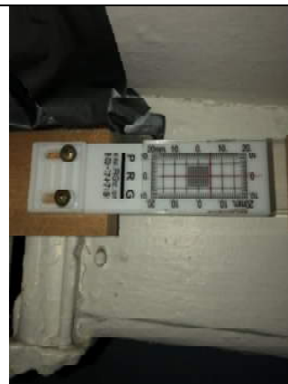
12) Current reading of crack monitor during observation.
