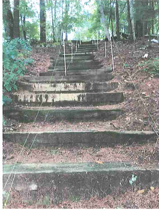
Steps to be replaced (facing Shore Drive)
