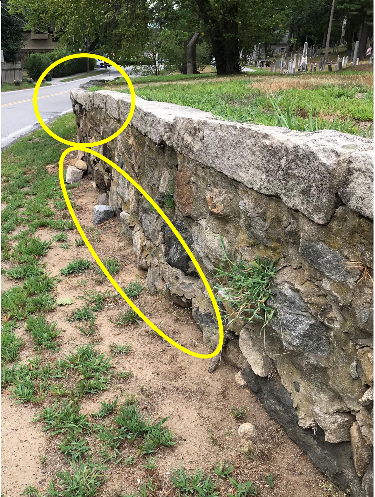
Figure 6. Retaining stone wall designated for reconstruction Location: 3-2 [cemetery boundary along Bedford Street] Issue: multiple stones dislodged; wall is leaning towards street
