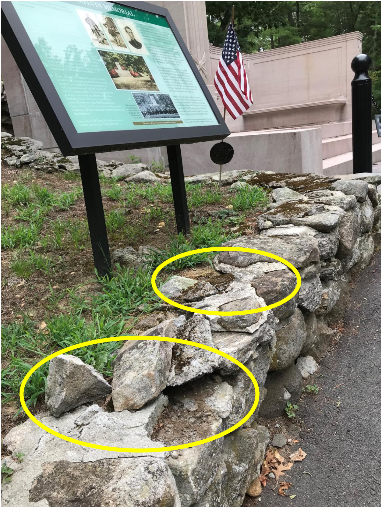
Figure 4. Retaining stone wall designated for reconstruction Location: 3-7 [Upland Ave, left of Melvin Memorial] Issue: multiple stones are dislodged/loose
