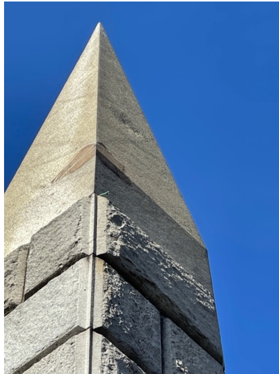
Close up top of monument – damage on corner that looks like it was repaired once and one of the pins – Photo by Beth van Duzer
