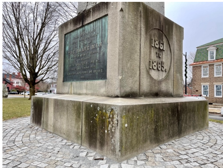
Base of monument with biological damage and the western tablet – Photo by Beth van Duzer
