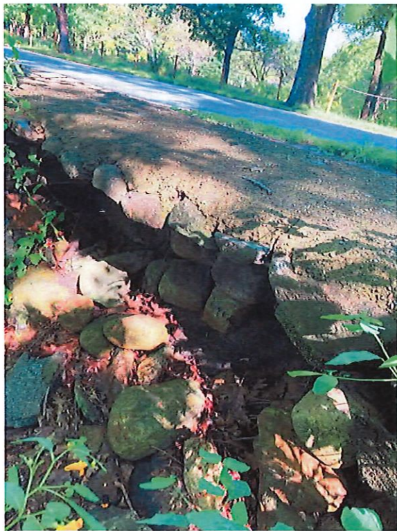
Figure 2: Failure along back side of wall
