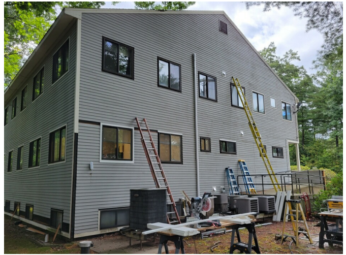
Facilities Division completes repairs to trim and clapboards at 37 Knox Trail prior to painting.
