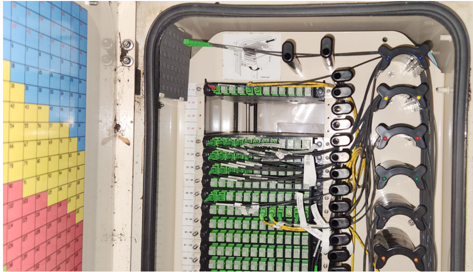
Figure 1: Local Convergence Cabinet (LCC)
