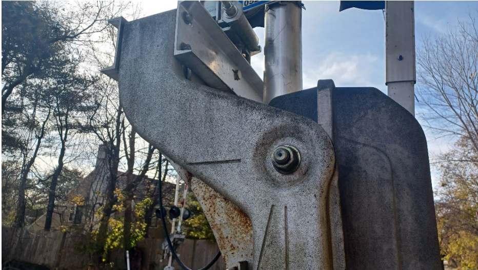
Photo 9: Deteriorated gate mechanism housing
