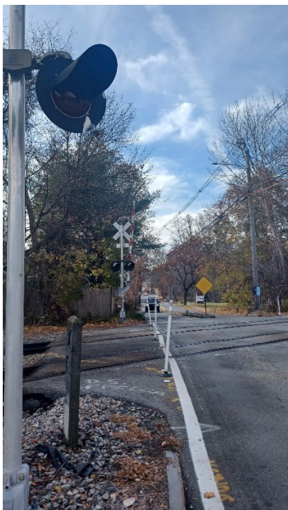
Photo 10: Signal light background on northeast quadrant, showing damage from vehicle impact, proximity to road
