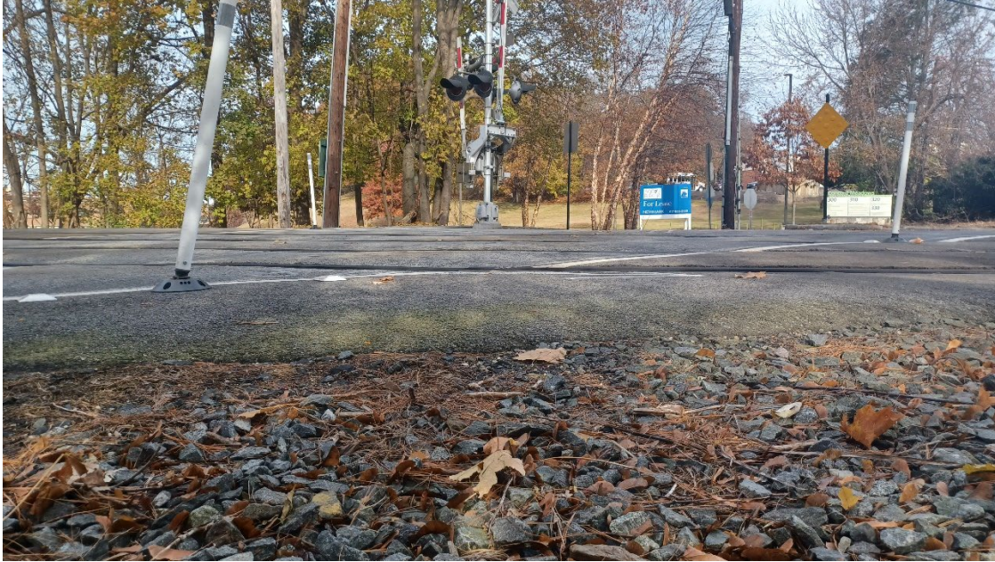
Photo 3: Settled roadway surface within crossing island
