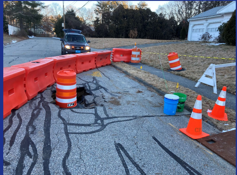
Sinkholes on Ministerial Dr
