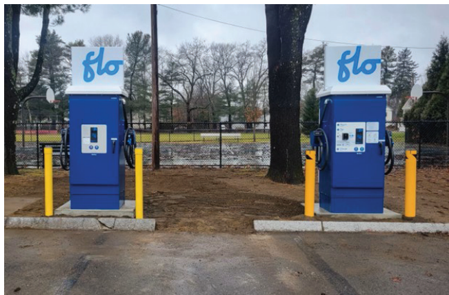
Level 3 Electric Vehicle Charger
