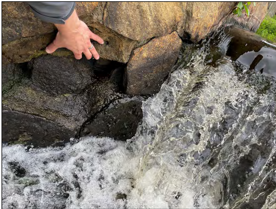
Photo No. 16.: Location of missing stone in right training wall
