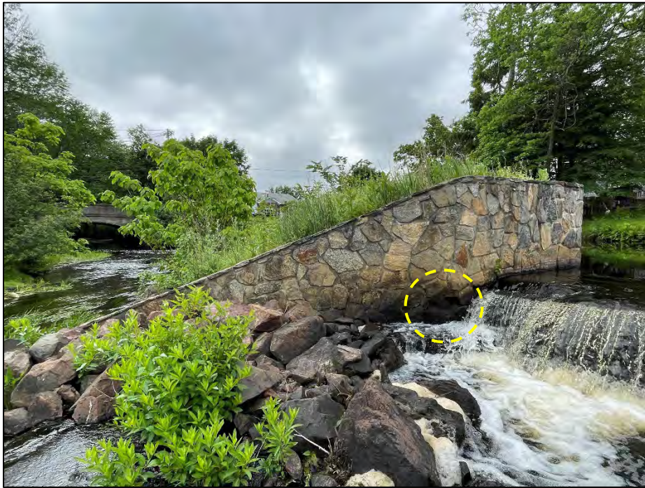
Photo No. 15.: Right training wall of primary spillway. Note the location of the missing stone and the leakage through one of the masonry joints
