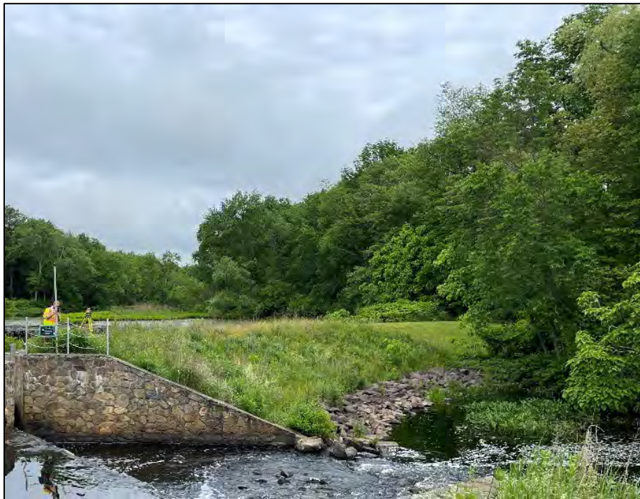
Photo No. 6.: Downstream slope from the embankment between the spillways looking left.
