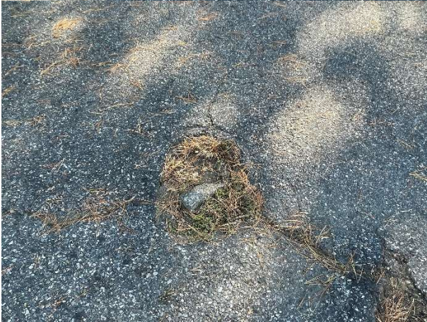
Details of damage to drive.
