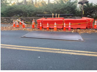
Baker Ave Culvert Collapse.jpeg
