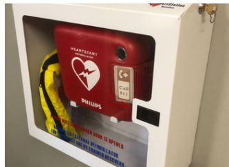
Defibrillator deployed in cabinet
