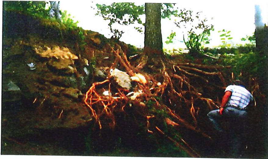
Tree root induced scouring on crest and downstream face of Coffey dam in Kansas
