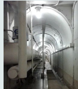
ISU steam tunnels
