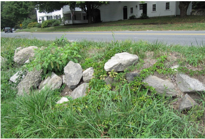
Deteriorated stone wall along Lexington Road
