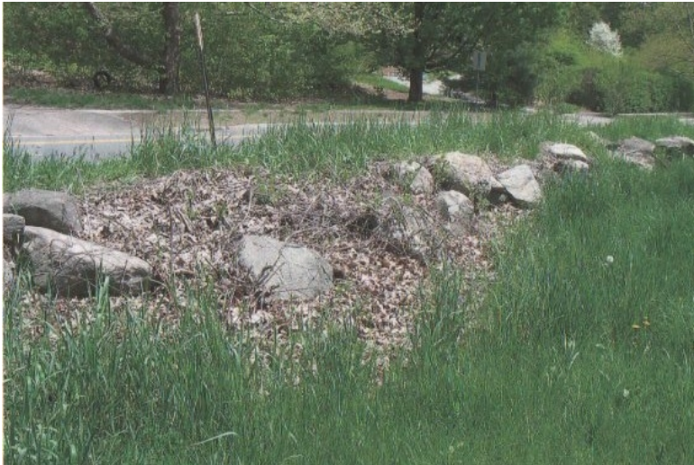
Deteriorated stone wall along Lexington Road
