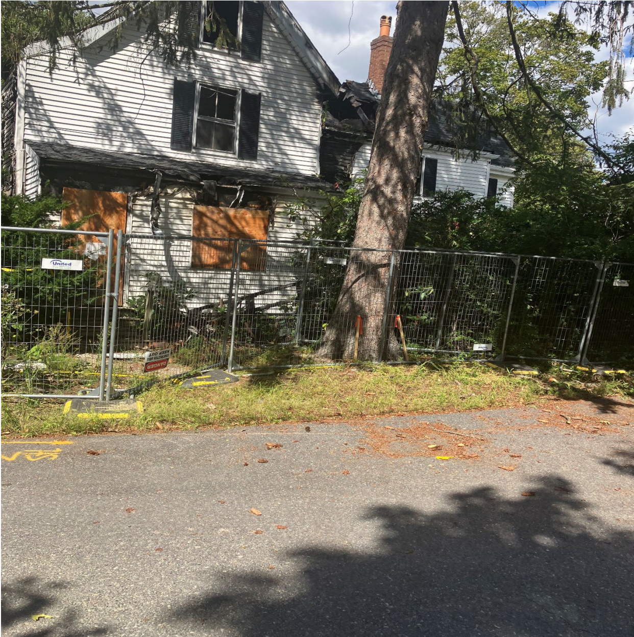
Photo of 24" Norway Spruce at 36 Cottage Lane prior to demolition showing proximity to street and structure.
