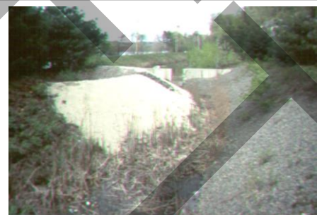
Filter berm acting as outlet for a detention area
