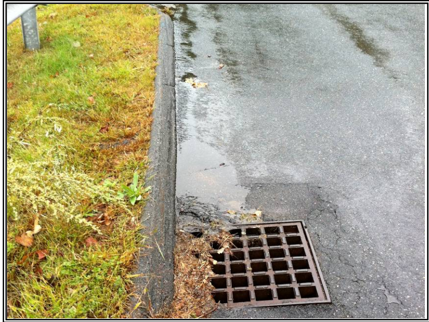
Photograph No. 9: Stormwater flowing into catch basin
