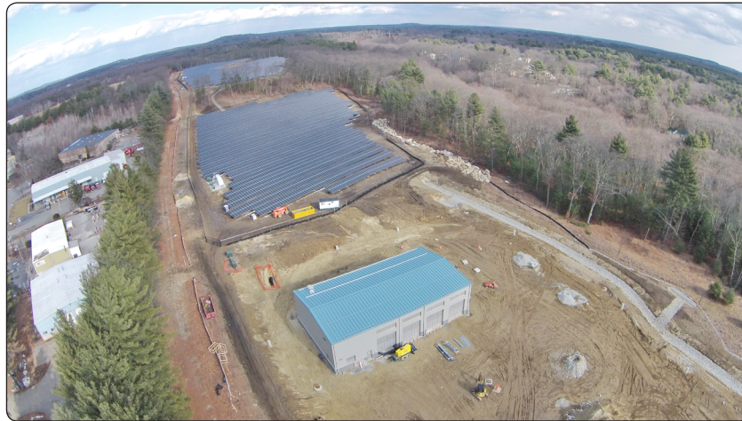
Aerial photograph of the new solar field off Knox Trail
