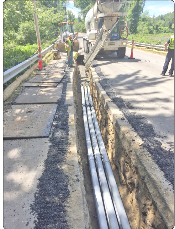
CMLP staff extended underground electrical and telecommunication infrastructure to the new solar site in Concord.
